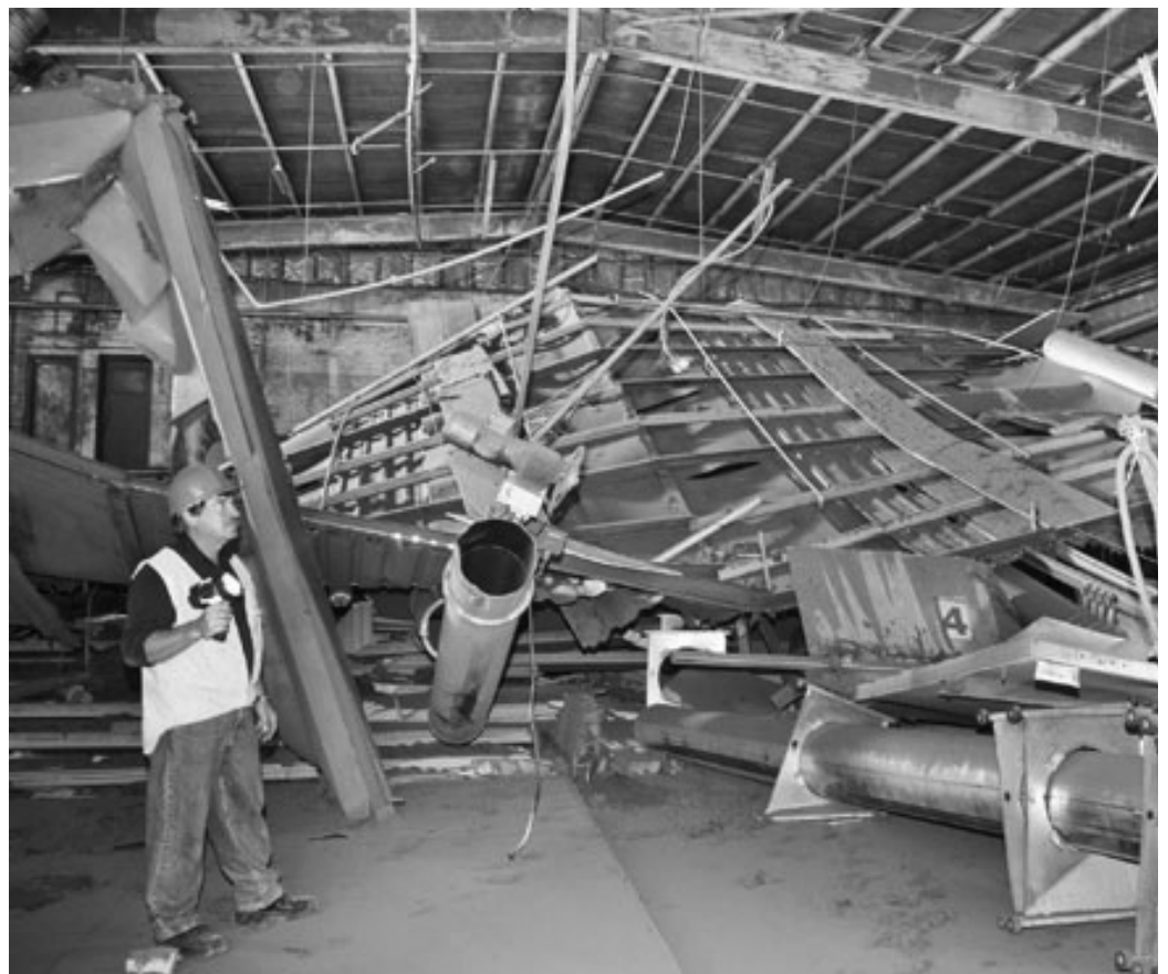
The Canterbury Spinners plant, which collapsed during the earthquake. 195 workers have since been made redundant.
